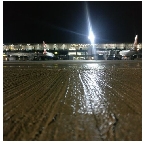
Fig 6- Slab after treatment
