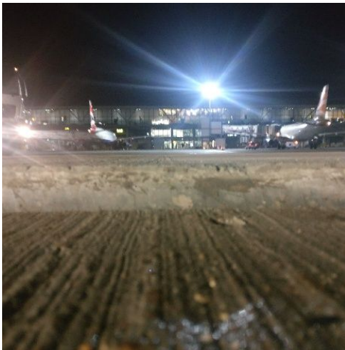
Fig 5- Slab before treatment
